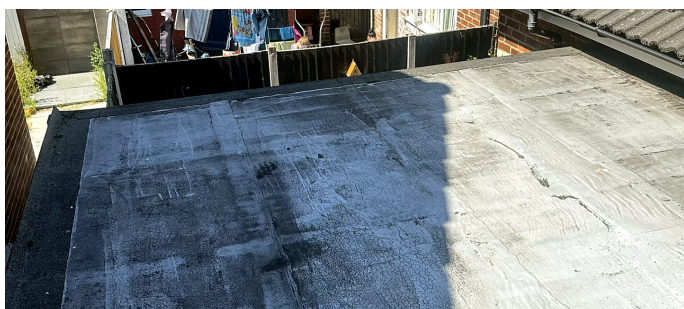
14 July, survey visit. Old felt, patched and ponding.
